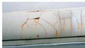
Cracking, due here to the filler beneath the paint lifting.
